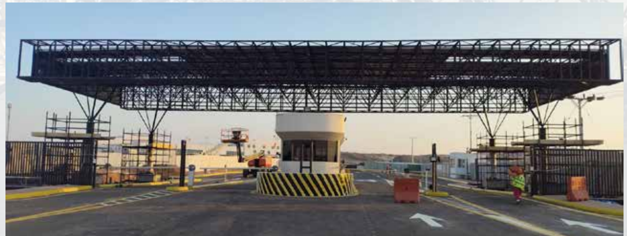
NEOM Community 2 Security Gate Sunshade
